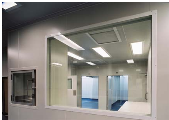
Class 7 cleanrooms with Vilair-AAF filtration system
